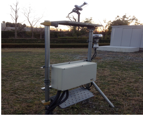
Figure 4.16: Sensor for measuring outside temperature and solar radiation.
