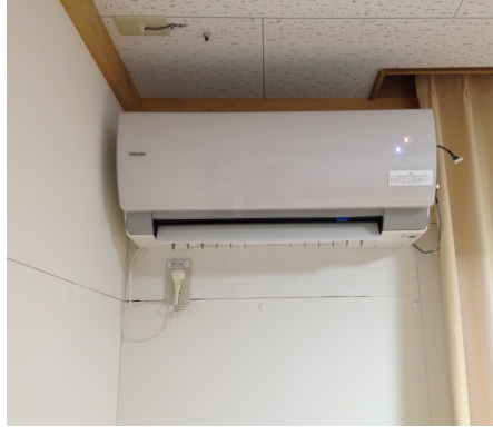
Figure 4.12: Air-conditioner mounted with sensor.
